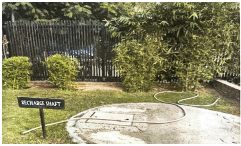
RAINWATER HARVESTING SYSTEM AT MRU
