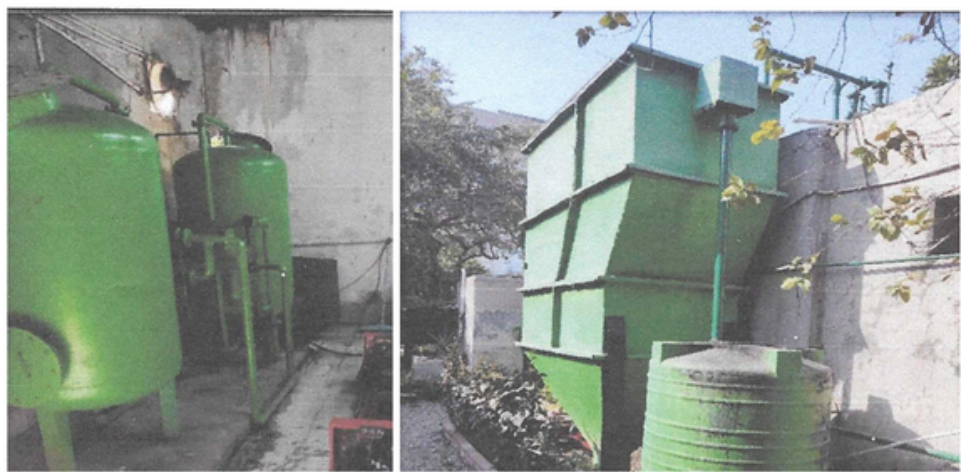
FILTRATION ASSEMBLY AND REACTOR TANK
