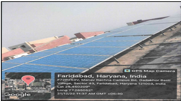
Solar Panel (Roof Top K-Block)
